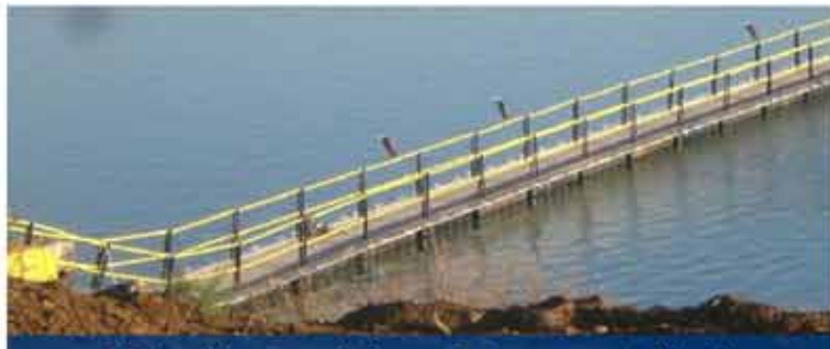
417m with pump platforms & pipe support Algeria
