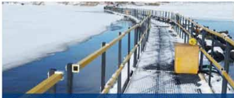
Dredging walkway with cable tray and ice grating
